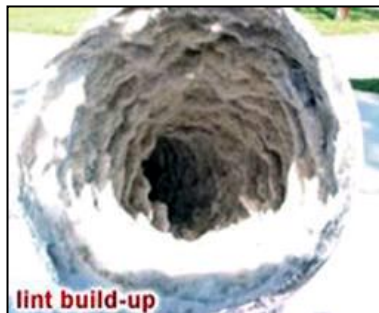
EXCESSIVE LINT BUILD UP
